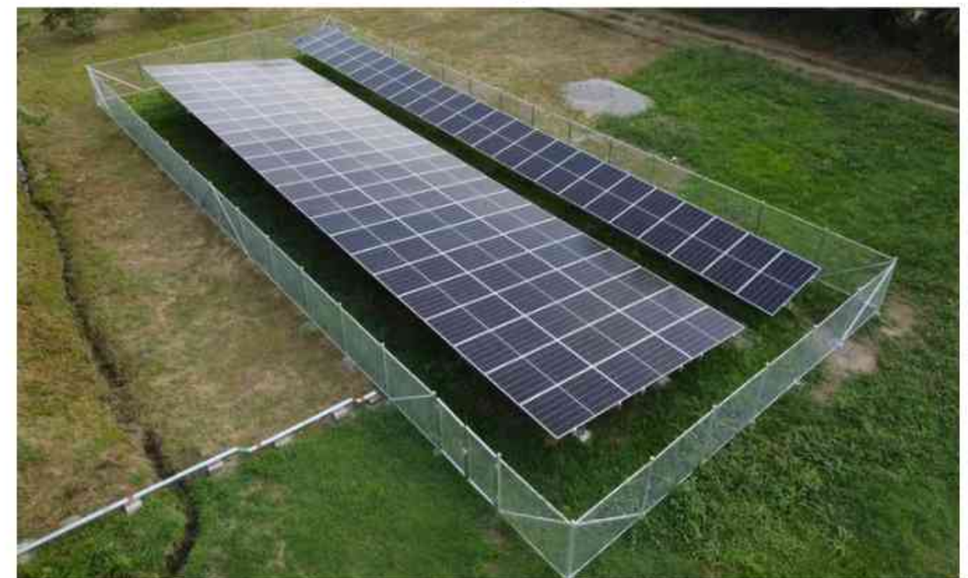
Sinefi - 90 paneles - 49.5 Kwp - Ibagué Tolima
